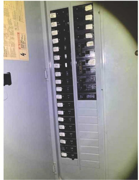
Breaker Panel At Garage
