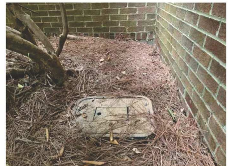
Water Meter and Exterior Cut-Off
